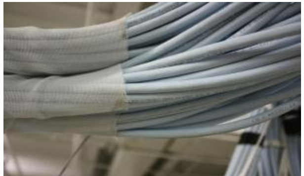
Fifty-Four (54) CAT 6A cables exiting Self-Supporting MaxCell
